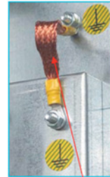
Bonding conductor between QEG and electrical pre/post-heating kits
