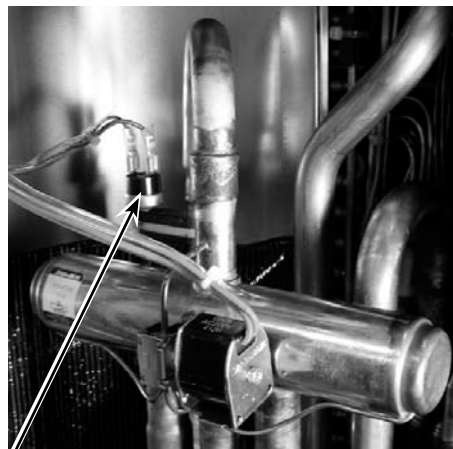
High pressure switch
