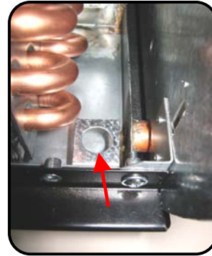
Condensate sensor fixing bracket at RH end of drain tray with grommet removed to give 13mm hole
