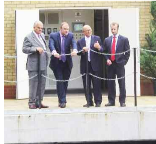
Secretary of State, Edward Davey, MP, visited the specially-built plant room adjacent to the river, which extracts heat from the river water without harming wildlife.
