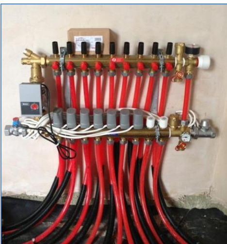
BELOW: The UFH manifold.
