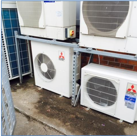
ABOVE: Smaller split air conditioning systems provide comfort to the mobility shop at street level.
