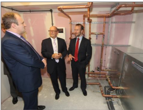
BELOW: Donald Daw (right) and Mike Spenser-Morris (centre), explain how the heat pumps deliver heating and hot water to the Edward Davey.
