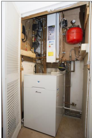
Below: Ecodan is efficiently providing 70% of the family heating needs.
