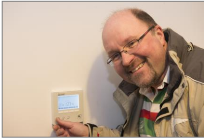
Above: Mike Newby has full control of his hybrid heating system through the simple wall controller.
