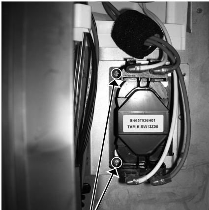
Screws of the reactor
