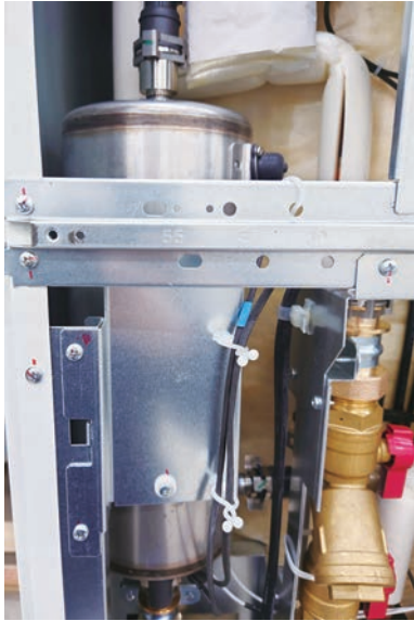
Photo 16-14-1 Booster heater assembly
