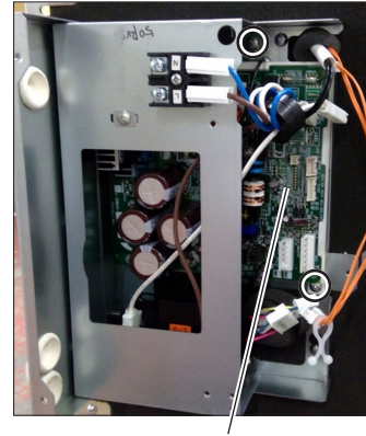
Power circuit board
