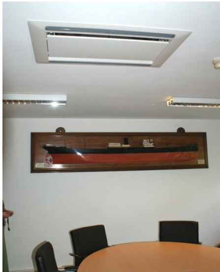
The ability to use existing pipework saves on installation time and costs
