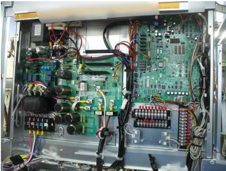
Air to water unit
