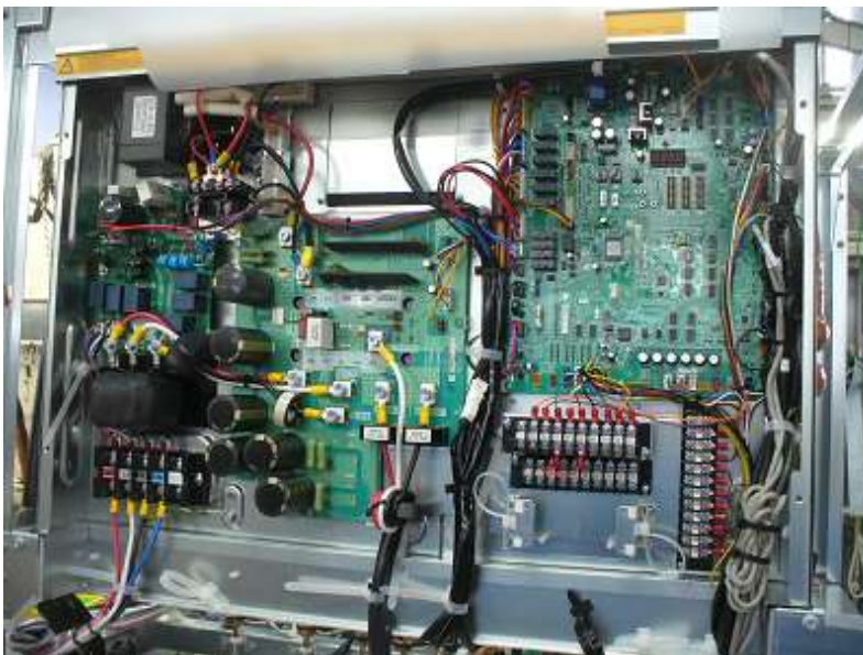
Air to water unit
