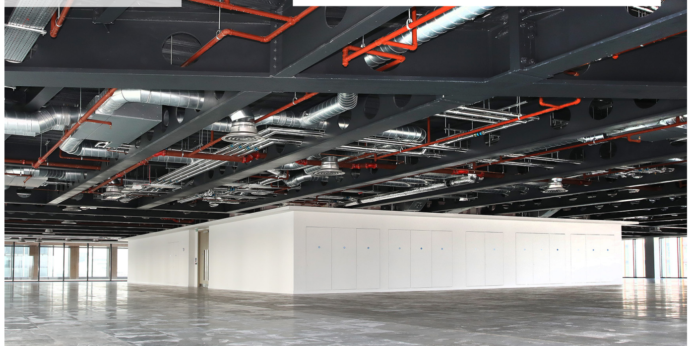
The exposed building services prior to the office fit-out
