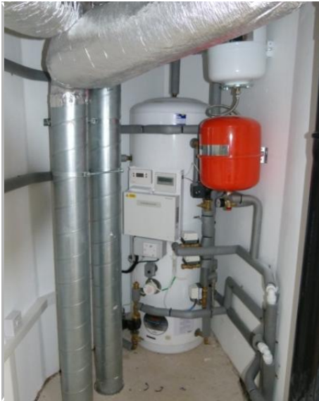
The Ecodan units connect to a water cylinder located in a specially-built plant room.
