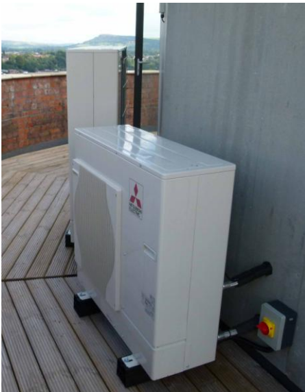
The Ecodan units are discreetly sited on the roof top.
