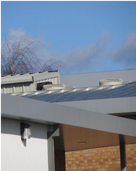
Air to water heat pumps have been discreetly sited on the roof of the new school building.
