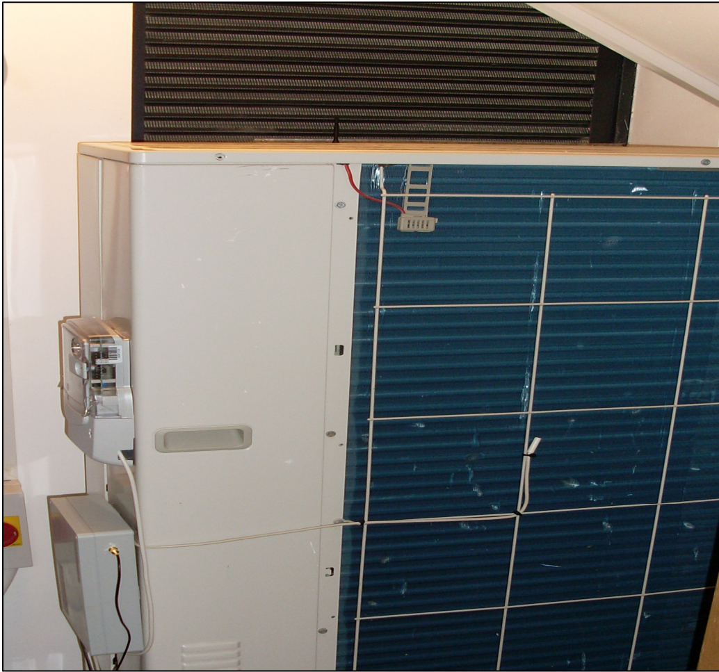
[Left Photograph] PUMY Outdoor unit housed inside the louvered enclosure.
