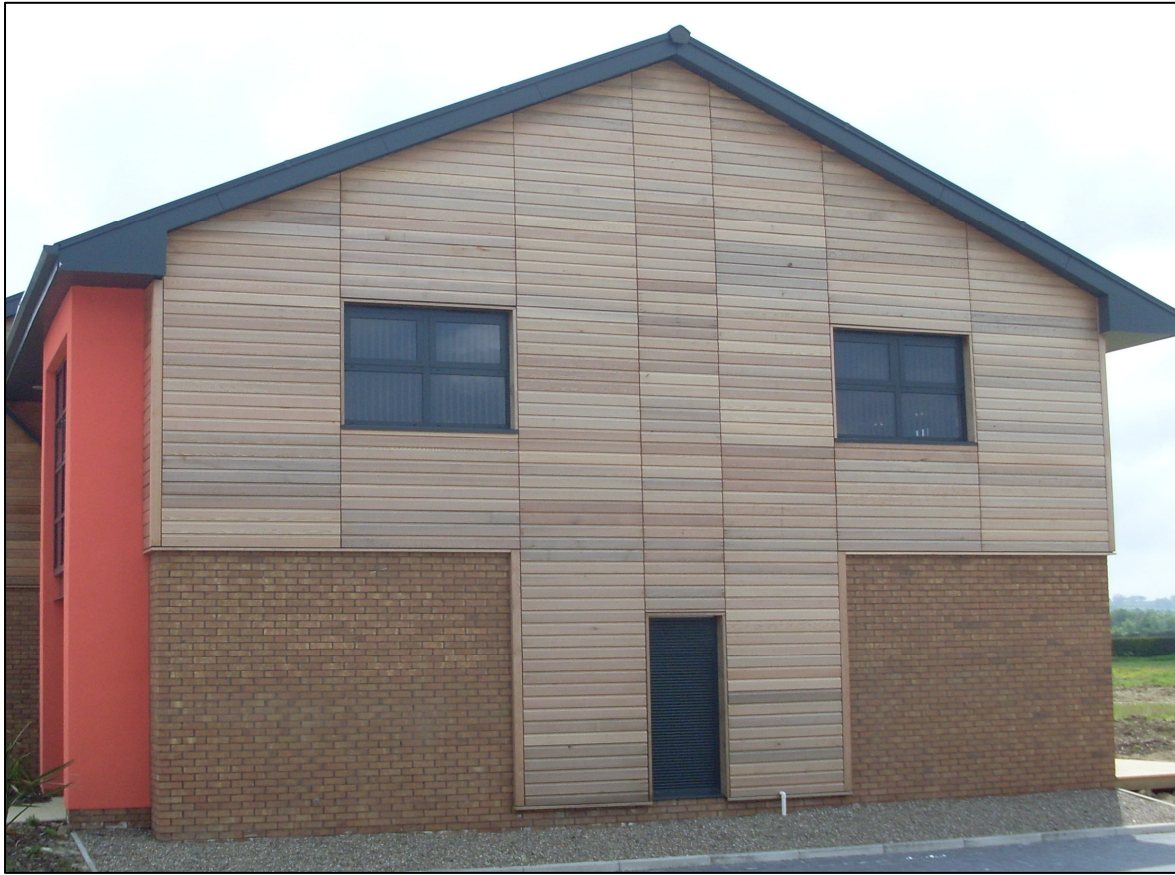
[Left Photograph] Shows the outside of the Louvered compartment in which the unit is installed behind.
