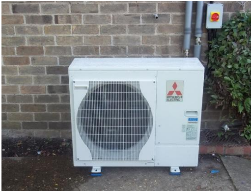
The 5kW Ecodan (PUHZ-W50VHA) air source heat pump fitted to the bungalow works at variable capacities between 1.5kW and 5.2kW.
