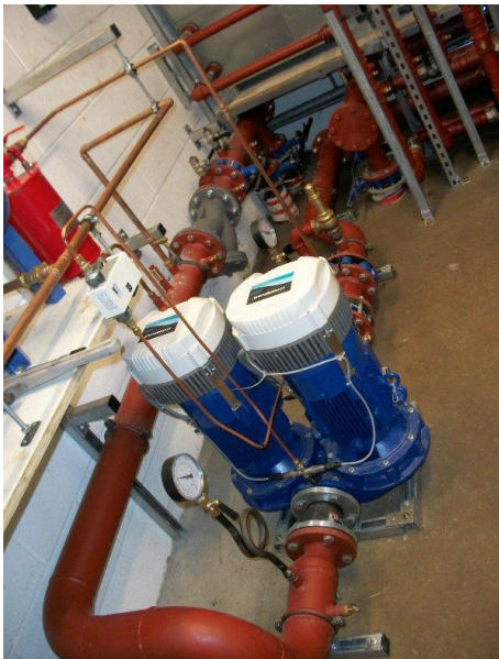
Circulation pipework and pumps to connect the groundworks to the heat pumps have been installed in the plant room.
